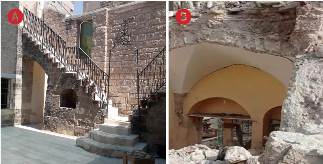
Heritage and Conflict in Gaza, Fig. 4 Al-Saqqa Palace: (a) Before the destruction. (b) After the destruction. (Photos by Hani Abu Riziq. These images have been
